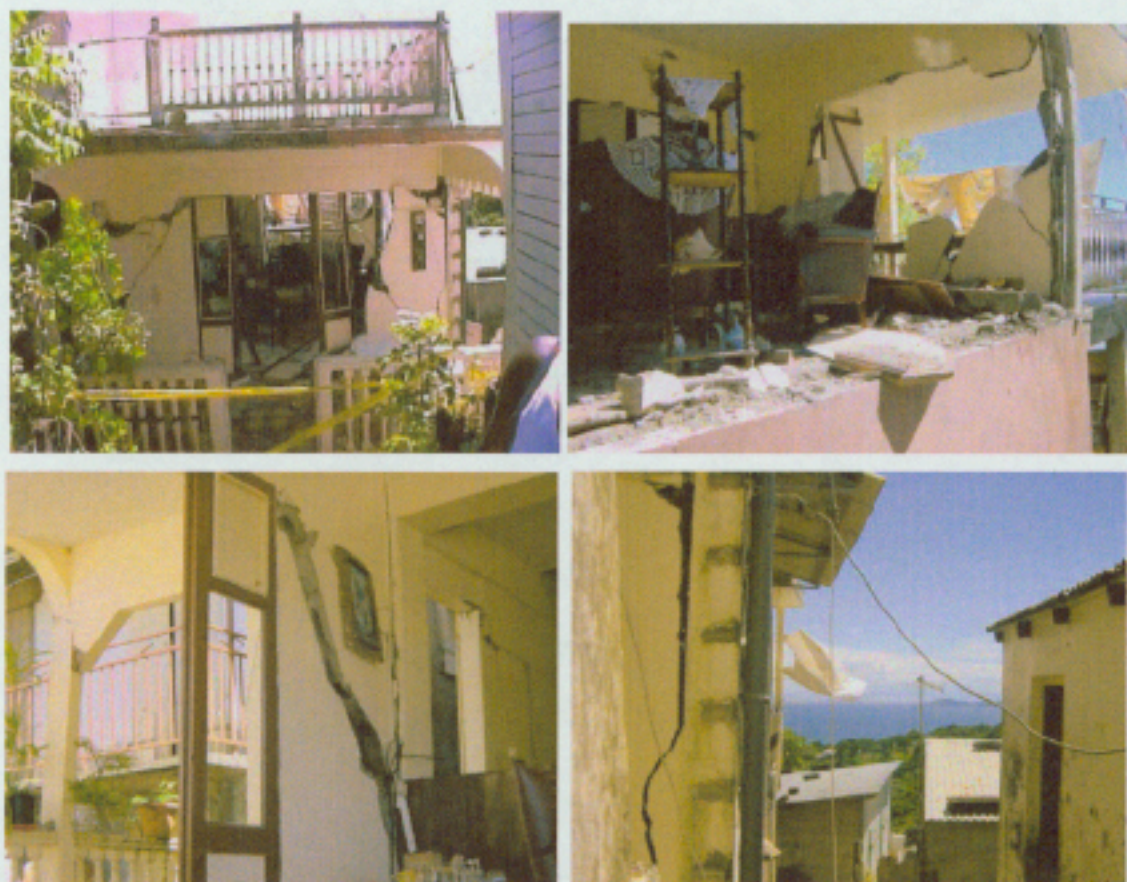
Figure 2. Houses at Trois-Rivières, Guadeloupe damaged during the earthquake (Photographs by N. Zahibo and A. Yalçiner). In the last photograph, the islands of Les Saintes, where the earthquake was destructive, can be seen in the background.
