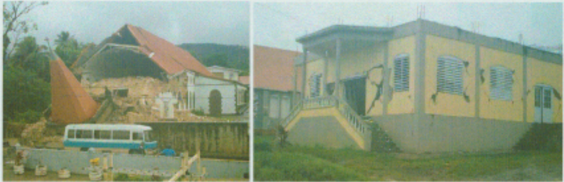
Figure 4. Roman Catholic and Methodist Churches at Portsmouth, Dominica damaged during the earthquake (Wayne Abraham, http://dominicapsn.freeyellow.com/gallery.html ).
