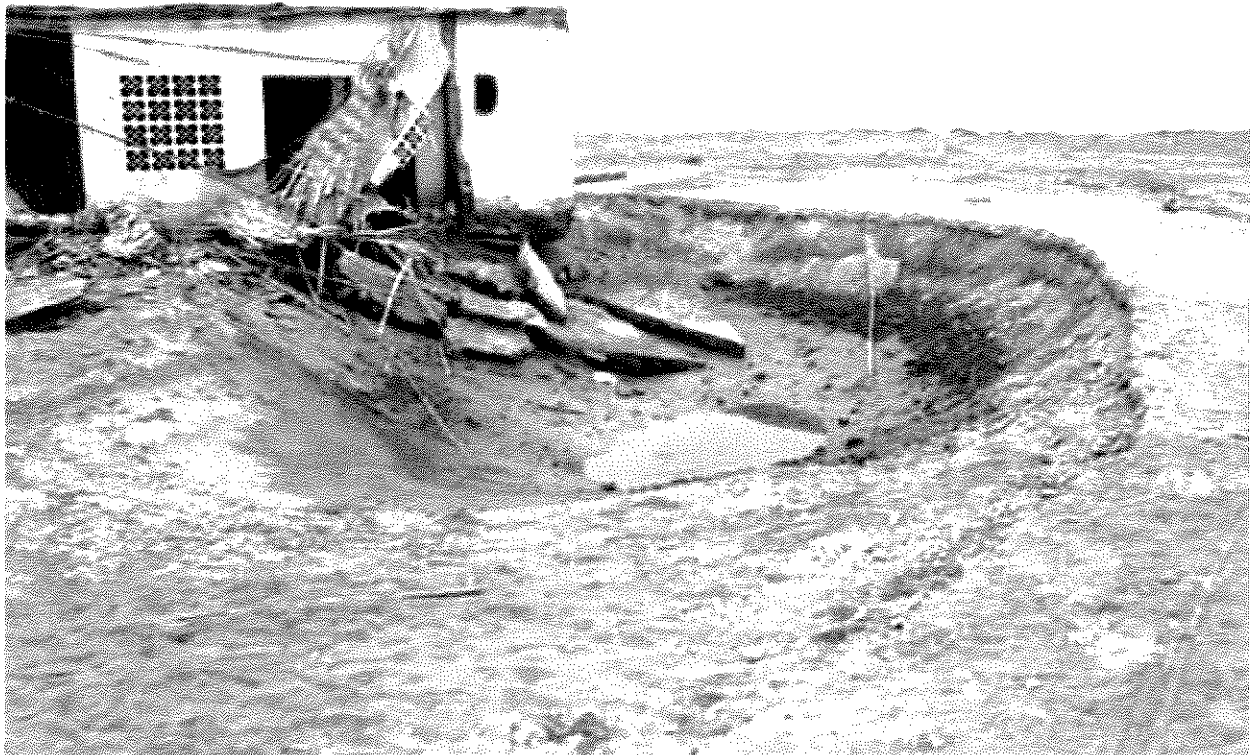
▲ Figure 10. Scour around the southwest corner of a La Punta house. Scour was observed at the corners of almost every structure in the inundation zone and next to paved roads.
