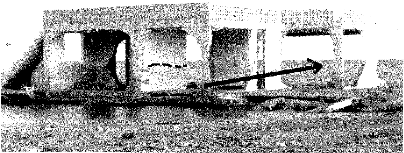
▲ Figure 9. Damaged summer home, La Punta. Typical construction consists of reinforced columns on a 20–30-cm-thick concrete slab foundation with unreinforced brick-infilled walls. Walls perpendicular to the direction of the tsunami (black arrow) failed. Dashed line shows a stagnant water mark.
